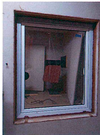
From source room side
