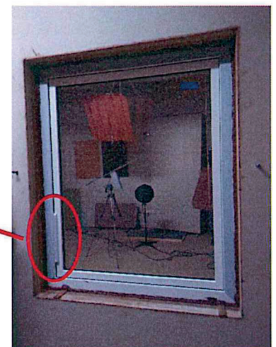
From source room side
